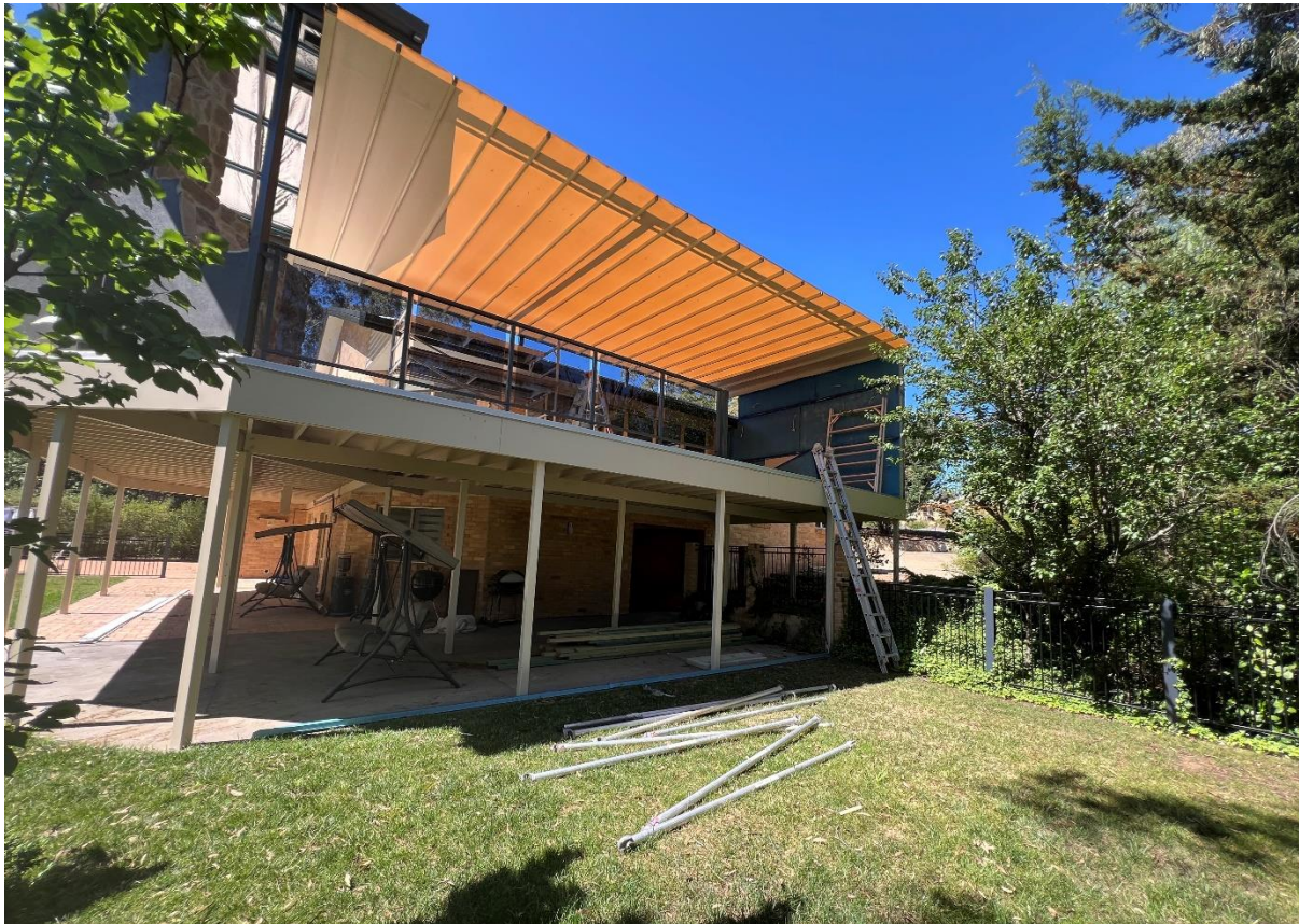
Figure 4: View of the existing retractable roof that is subject of a separate BIC application
