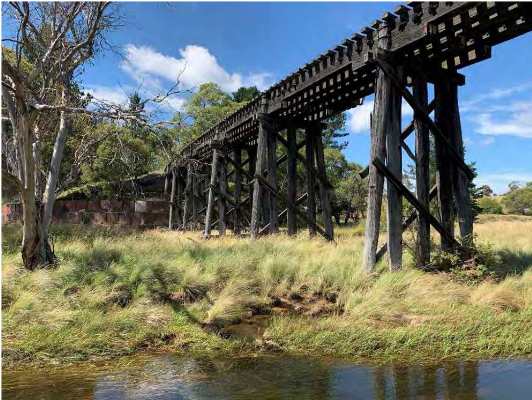
Figure 10-1: General view of MacLaughlin River Bridge from abutment 2 looking towards abutment 1. The timber bridge is 8 spans long and approximately 60 metres in length (7.5-8m spans). Note MacLaughlin River runs underneath span 3 and is approximately 3m wide and 0.7m deep. It was also noted that the bridge curved left and had appropriate camber. Note the double cross bracing on the bents as well the absence of a sash brace.
