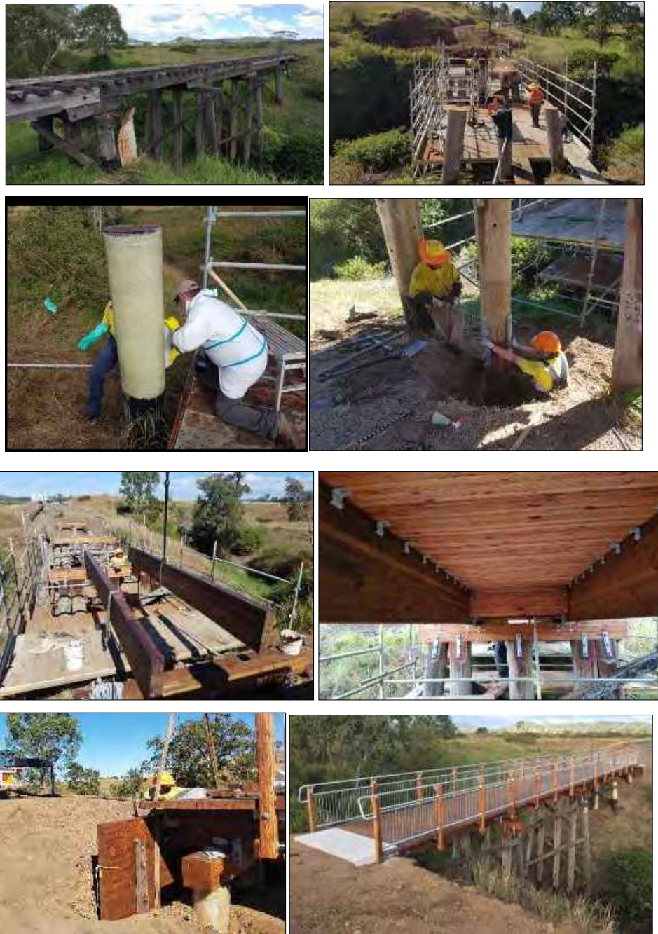
Figure 12-4: The photo series above demonstrates Option 3 type of fix that was completed on Jimmy Gully Bridge along the BVRT. The existing poor condition superstructure was removed, and the piles were repaired with high strength fibre or posted with new section. New glulam back wall, caps, girders and deck system were installed utilising a horizontal connection detail.
