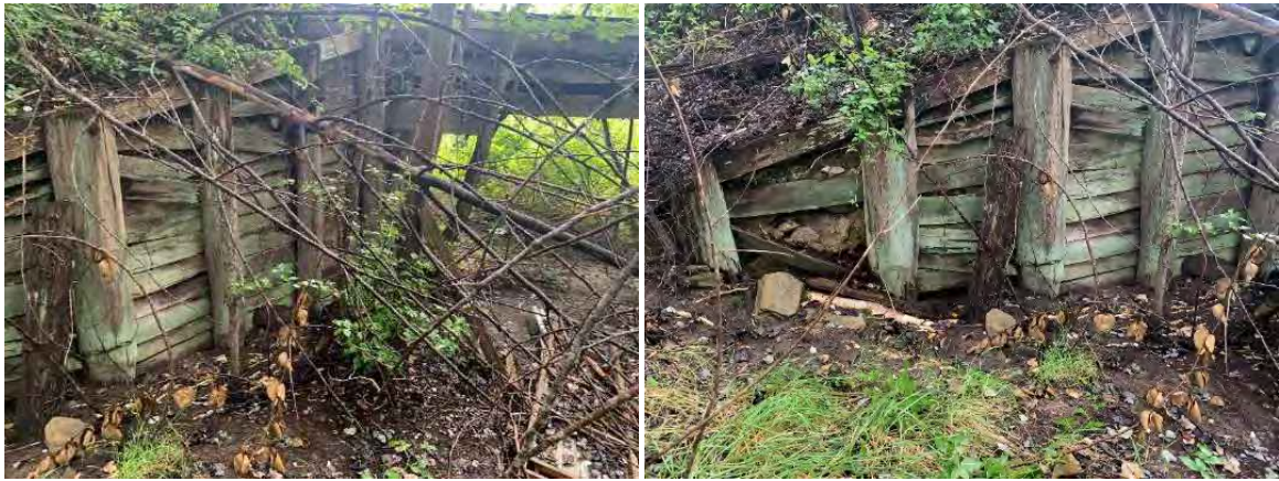
Figure 4-8: The timber wingwalls have undergone significant deterioration with timber sheeting completely rotted and failing in several locations. Due to this the walls' ability retain the approach fill material is poor leading to erosion and excessive loading.
