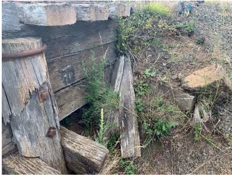
Figure 11-5: View of abutment 1, found to be in poor condition with major decay of sapwood present in piles and broken/missing elements in abutment sheeting.
