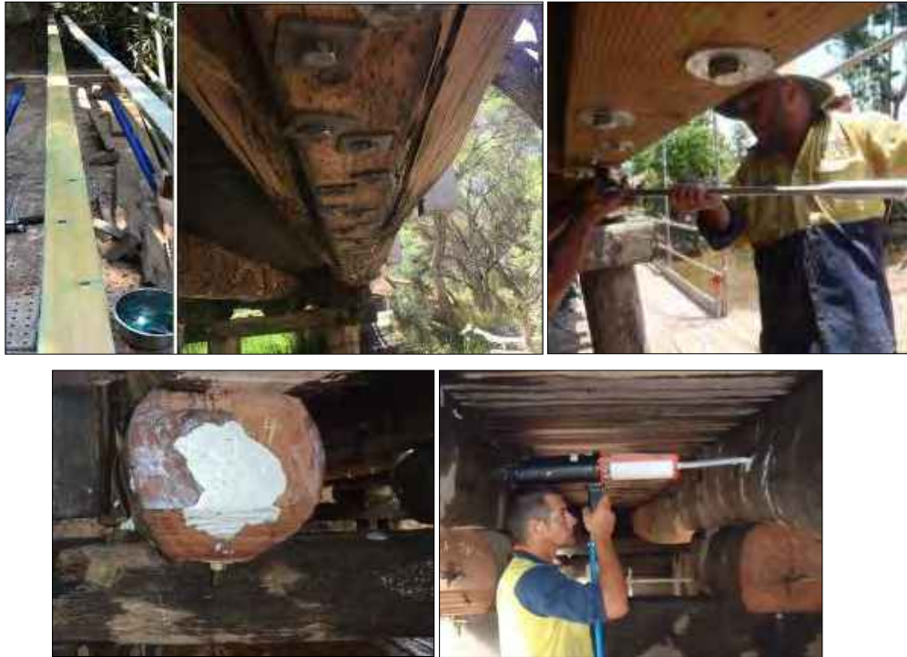
Figure 12-5: The repair of Meachams Bridge in Cassowary Coast. The bridge was retrofitted with fibre reinforcement on the bottom of the girders, some corbels and girders were injected with a high strength epoxy. Some piles were also wrapped with high strength fibre and injected with epoxy, then the entire bridge was diffused with borate salt rods to neutralize decay growth.
