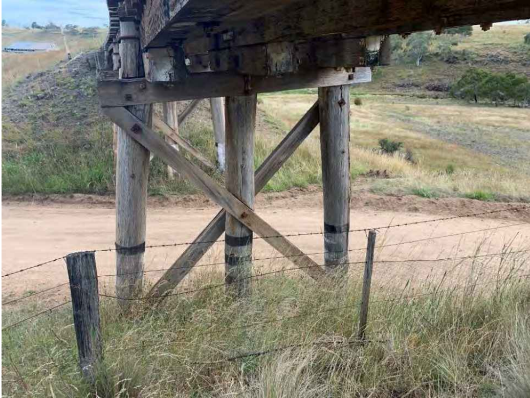
Figure 11-2: View of pile bent 1 configuration. The bents comprise of 3 driven piles. Pile bent 2 and 3 are supported by cross bracing. The two abutments do not contain the cross bracing but are supported by sheeting planks to retain backfill. It was noted that several piles and headstocks have started to undergo decay. It can be seen on pile 3 significant sapwood decay occurring.
