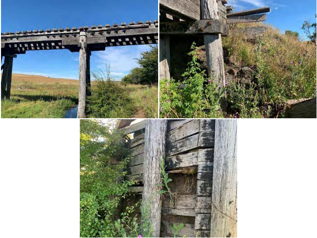
Figure 9-5: Large amounts of sapwood decay is present throughout the structure piles. It is recommended that this is monitored and removed appropriately.
