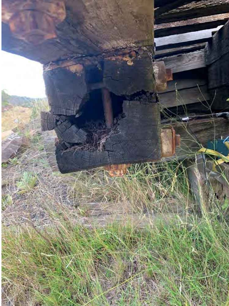
Figure 11-9: View of corbel 3 at abutment 1, Corbel was found to be in very poor condition with a large cavity present in the end. The vertical connection is visible highlighting the depth. The corbel needs replacement due to multiple failure points. Note the vertical fastener has split the corbel and the anti-splitter bolts have done the same thing. So many of these old details contributed to higher maintenance costs and reduced longevity.
