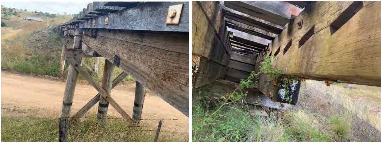
Figure 11-6: A view of girders formation and condition. Girders were found to be in fair to poor condition, the left photo shows a horizontal crack that is seen to be progressively increasing in size. The right photo shows sapwood decay of the internal girders.
