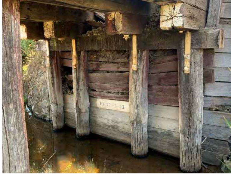
Figure 6-4: General view of Abutment 1 shows the timber sheeting in very poor condition as top half is failing and backfill material is eroding. Note: Hole in decking above abutment causing significant material loss from rock ballast above.
