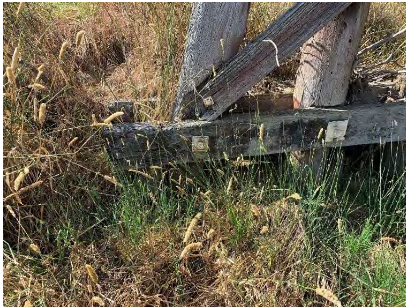
Figure 8-6: A view of a cross bracing plank connection. Plank was found to be in very poor condition as the end has completely decayed away to the connection point. Timber wales were found to be in poor condition with significant water stains and decay present throughout.
