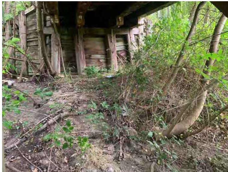
Figure 4-3: Both abutments consist of 4 timber piles, timber headstock, timber corbels and timber sheeting. It was noted that the bottom section of several piles has started to undergo decay. Note abutment sheeting is rotted and failing. Timber pile and sheeting wing walls present on both sides of each abutment. Once the moisture content in the timber elements reaches 22%, decay causing fungi are activated and the decay process begins. Large trees need to be cleared as their root systems apply lateral pressure on the substructure elements as will the branches and trunks on super structure elements.
