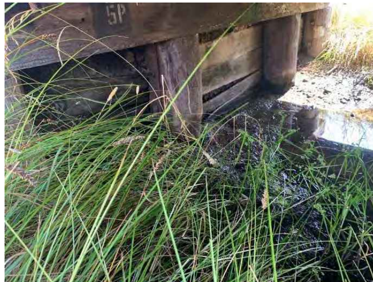
Figure 7-3: View of abutment 2, overall, in a poor condition. Sheeting planks have separated due to spiking to the pile backs in the breast wall, causing loss of fines in the approach fill material through gaps.
