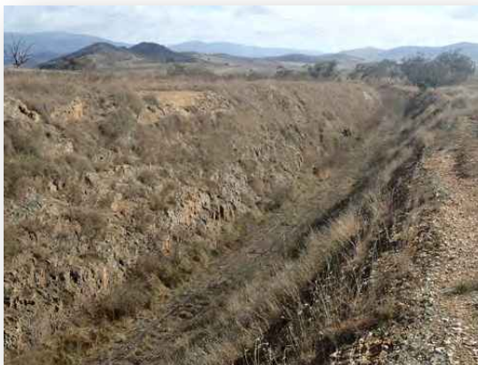
The old drains of the many cuttings along the proposed rail trail will require attention to ensure they still perform the task of clearing water from the cuttings
