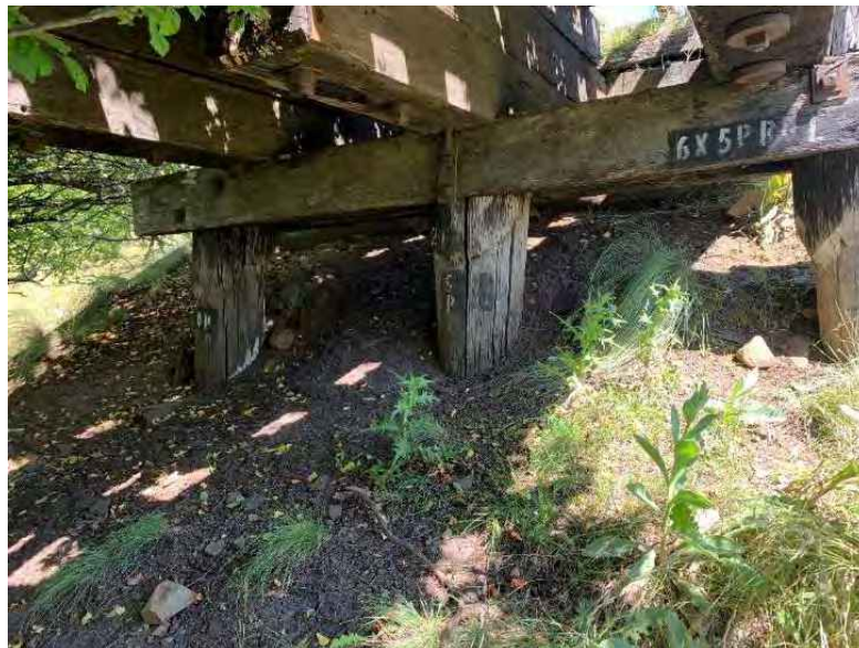
Figure 10-8: View of abutment 2 configuration, the abutment was found to be in poor condition with significant decay present. It was noted that the left two piles had large vertical splits in them, whilst the right pile had significant decay of sapwood.
