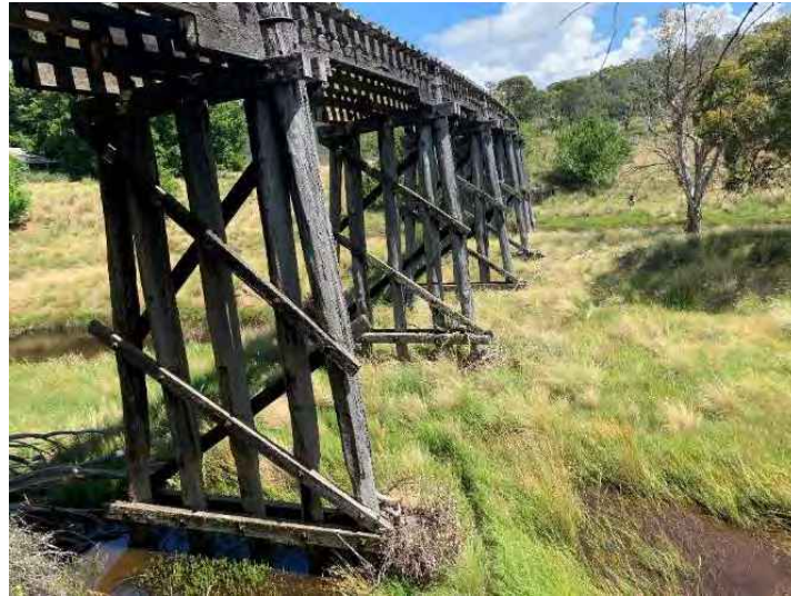
Figure 10-7: Above image shows the left curve and camber in the bridge. The bent configuration is also highlighted, it was noted that significant overgrown vegetation and debris build up was present at the base of all bents. This increases moisture retention leading to accelerated decay of the lower timber elements.
