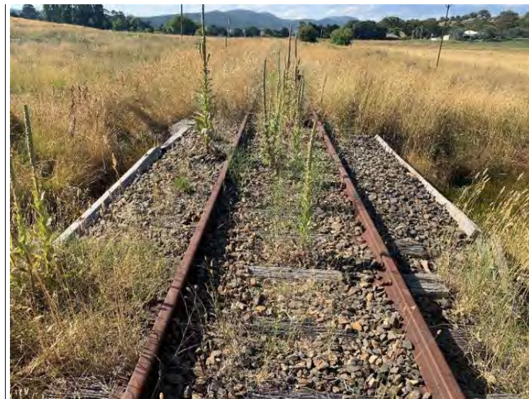
Figure 7-7: The photo above shows the general view down the rail line. Significant overgrown vegetation present through rock ballast and surrounding the substructure. Note: Ballast is 450mm thick.
