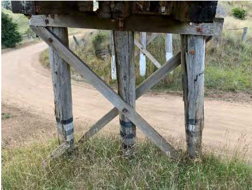
Figure 11-3: General view of pile bent 2. piles were found to be in poor condition. With significant sapwood decay present in all piles, it was noted that all piles have large vertical splits through the horizontal connections. The bottom sections of the timber piles were determined to be a ‘hotspot’ for decay due to increased moisture retained by the overgrown vegetation.
