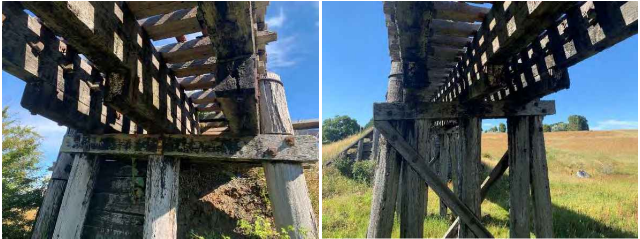
Figure 9-3: The images above show the substructure configuration. It is seen that double stacked girders have been used in addition to split headstocks and corbels. Both images show significant water stains and decaying of corbel ends. The left image identifies a large cavity present in the end of corbel 1 AB1. It was noted that AB1 sheeting has failed.
