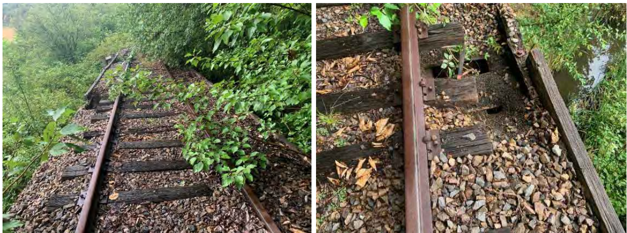
Figure 4-5: The timber transoms were found to be in a very poor (unsafe) condition. The timber ballast tray side walls and rock ballast were in poor condition with erosion of material found in several locations. If the bridge was to be repurposed for pedestrian and cycle use the timber transoms, railway line and rock ballast would need to be removed. Depending on the condition the existing ballast tray side boards they can left in place to act as a kerb/kick rail in the re-purposed bridge. To meet the current standards and Australian codes; vertical balustrade panels and a 1.4m high cycle rail will need to be installed. Note: Significant vegetation growth. The ballast tray will provide a great subgrade for the walking track.
