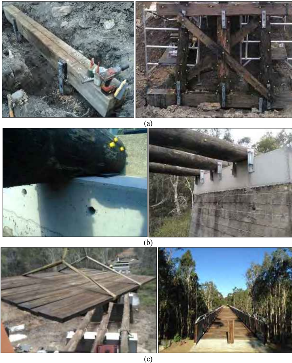
Figure 12-3: The above photo series demonstrates Option 2 type of fix (hardwood) used for the construction of two Mary to Bay Rail Trail Bridges. Seen above in photo (a) is the construction of a frame bent using an intermediate cap which was installed on top of the existing pile stubs. This allowed the hardwood posts, cross bracing, and cap to be installed at the correct reference height. Also note the yellow plugs that indicate that Decaystop® rods have been installed. Photo (b) shows the girders being installed using a horizontal connection system and a rubber liner between the timber girder and concrete pier. In photo (c) the pre-panelised deck is installed along with the modulus handrail and cycle rail system.
