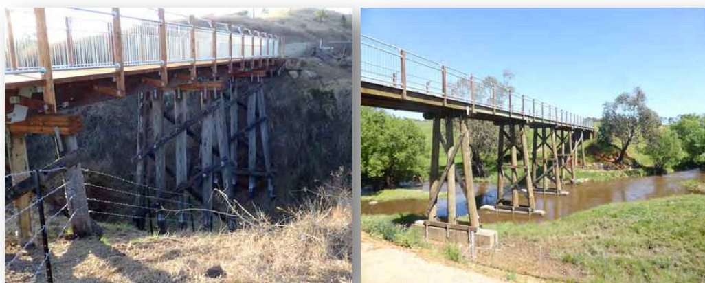
Renovating original railway bridges adds significantly to the trail user's experience. The bridge on the left is on the Brisbane Valley Rail Trail while the bridge on the right is on Tumbarumba-Rosewood Rail Trail. Both are restored in accordance with designs by WRD and both are good examples of restored railway bridges. Both use a combination of old (existing) and new timbers.
