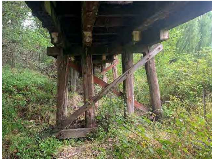
Figure 4-2: View of the typical timber pile bent configuration. The bent is comprised of 4 driven piles, single timber head stocks and corbels. The bent is also supported by a double cross bracing system with sashes at halfway and timber wales at the bottom. Overall, the timber bents were found to be in a poor to very poor condition. Note the surface brown rot fruiting bodies on the faces of some of the cross braces -orange brown colour.
