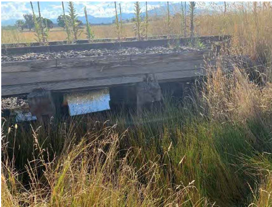
Figure 7-1: The image above shows a general view of the 7m minor bridge (Williamsdale Rd). The consists of 3 spans each span is 2m in length, substructure includes 2 pile bents and 2 abutments that each have 4 driven piles, a pile cap and 4 girders. At the time of inspection there was water approximately 0.5m deep in Spans 1-3. There is a large amount of vegetation growth around the substructure which keeps the moisture content high in the timber. When the moisture level in the timber is above 22%, decay-causing fungi can start to grow; when the moisture content drops below this level, the fungi become dormant, and decay will be arrested until the moisture content rises again.
