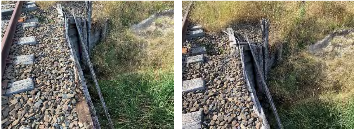
Figure 6-8: View of timber ballast tray side walls, spacing between side walls was 3.5m. Side walls were found to be in very poor condition with significant rot and decay present.
