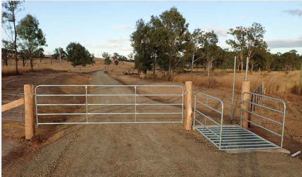
Above: a newly constructed management access gate and access grid on the Brisbane Valley Rail Trail (Qld).
