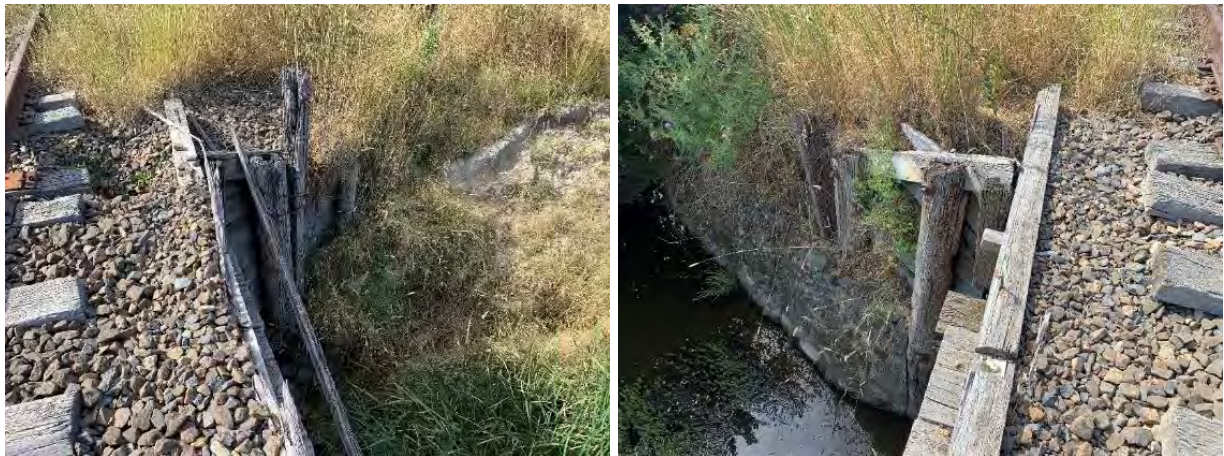
Figure 6-5: Above photos show the existing condition of the wingwalls. The wingwalls were found to be in a poor to very poor condition, multiple members had failed, and significant deterioration was present throughout.
