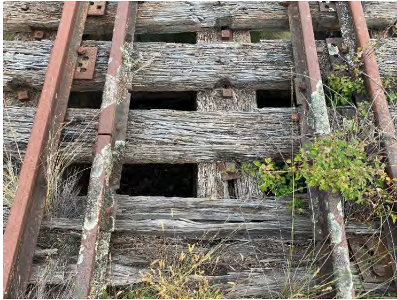
Figure 11-7: View of the bridge open deck, transverse sleepers were found to be in poor to very poor condition with significant decay, cavities and severely damaged members present throughout. It was noted that the vertical connections to the top girders were seen to funnel moisture and increase the moisture content present in both elements causes significant decay. When the moisture content exceeds 22%, timber consuming fungi are activated, and the decay process begins. Top girders were found to be in poor to very poor condition.
