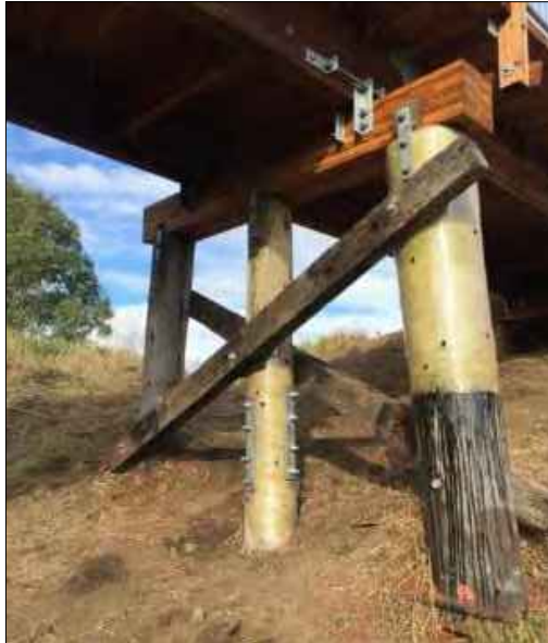
Figure 12-8: Diffuser (Borate Salt) rods are installed in the remaining hardwood elements to resist further deterioration of the timber caused by fungi growth. Note the red bungs are the decay ‘hotspots’ where the timber is prone to have a higher moisture content. These holes are required to be checked for rod depletion as per the issued maintenance manual (typically every 2-5 years depending on environmental conditions).
