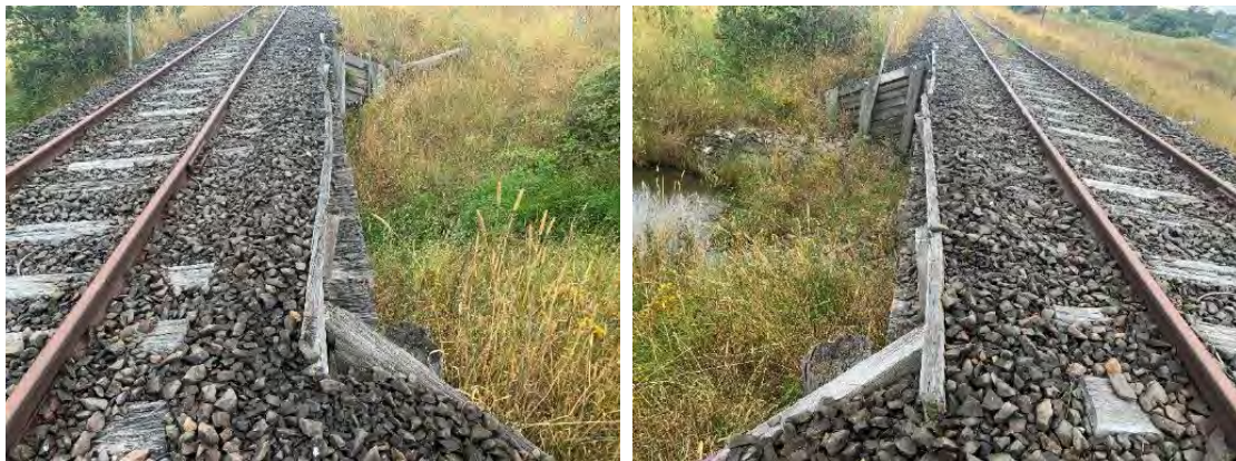
Figure 5-7: View of both ballast tray side walls. Both side walls were found to be in fair to poor condition, with minor deterioration of sapwood present at all lengths. Photo on the right shows the side walls support leaning backwards creating a deformation in side wall length. Photo on the left shows a significant bow in middle length due to bearing the load from the rock ballast.
