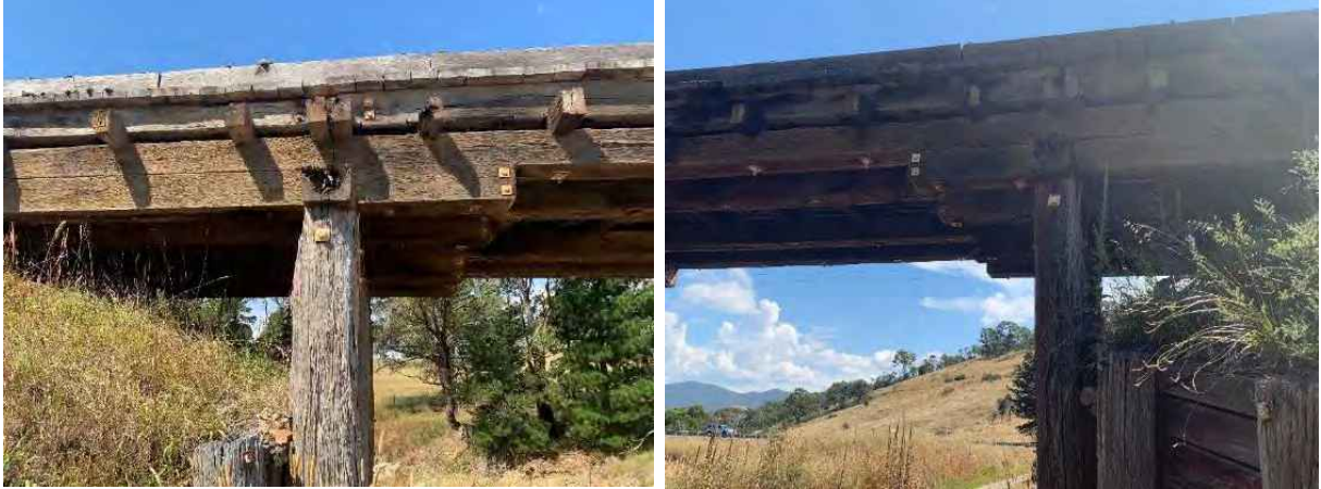
Figure 8-5: View of pile caps at PB1 & 4. Caps were found to be in very poor condition due to the significant cavities present in both ends of each cap. Note: The right photo also shows the backfill from PB4 pushing the breast wall forward.
