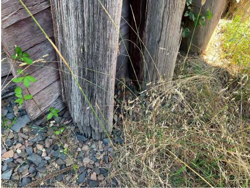
Figure 8-10: View of pile at PB4. Pile was found to be in very poor condition with significant decay present. Decay of approximately 50% of the cross section.
