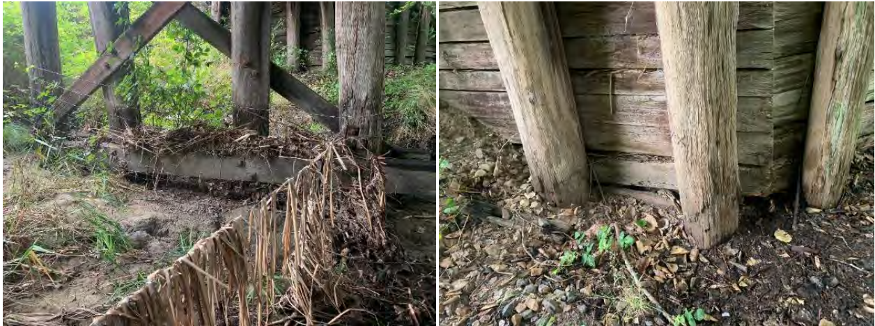
Figure 4-4: The bottom sections of the timber piles were determined to be a ‘hotspot’ for decay, this is caused by the moisture retained by debris increasing the moisture content in timber members. Sapwood decay in the timber piles is photographed on the right-hand side. Refer to Section 4.1 below for a full list of recommended repair options for refurbishment to a pedestrian/cycle bridge.
