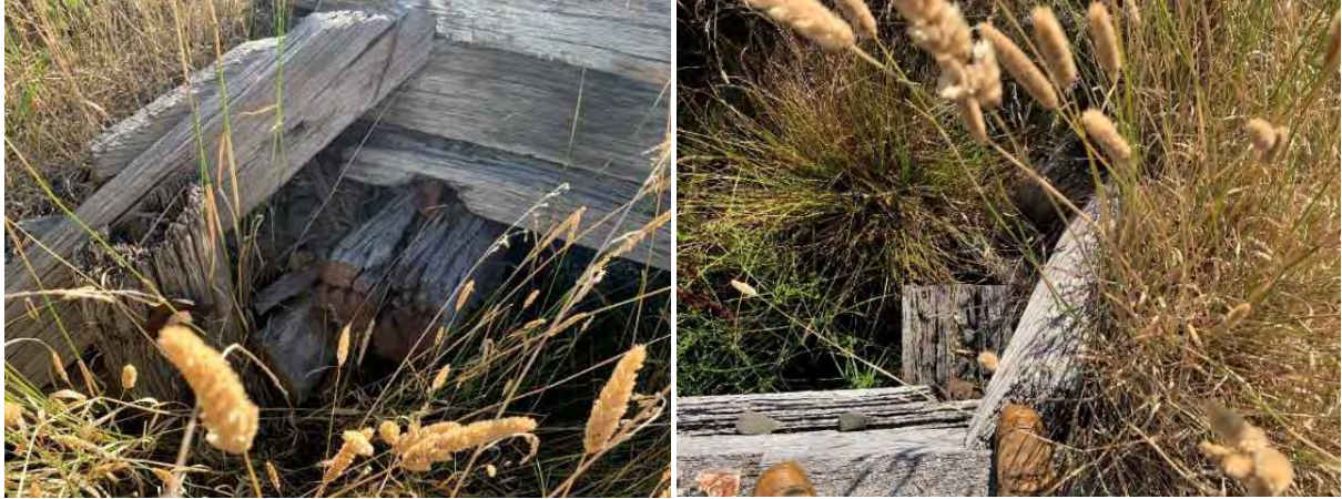
Figure 7-4: Top view of abutment cap connection. Cap is in very poor condition; severe deterioration is present in the ends and at the vertical connection. When a vertical connection is not sealed appropriately it exposes the heart wood to excess moisture accelerating decay. As seen in the photo a large crack is present at the end and a cavity is present at the top of the vertical connection.
