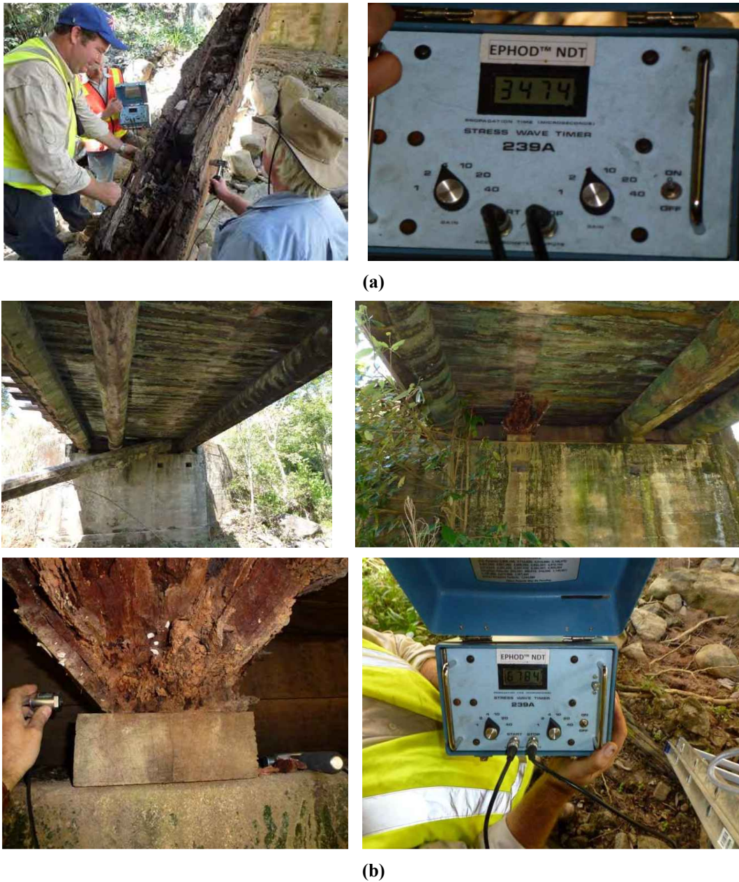
Figure 12-1: Photos showing global failure of a timber log girders. Both failures were caused by advanced decay in the ends of the girders and transverse shear failures. The primary cause of this decay was due to vertical fasteners. These failures were found in elements with SWT values in the 3k \mu s (photos a. above) to 6k \mu s range (photos b. below). Typically, similar bending extreme tensile fibre failures in log girders occur in zones of decay where there are over 2k \mu s SWT values. Similarly, if vast portions of the log girder have SWT values over 3k \mu s the failures may occur.
