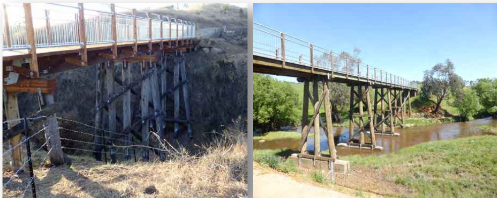
Renovating original railway bridges adds significantly to the trail user's experience. The bridge on the left is on the Brisbane Valley Rail Trail while the bridge on the right is on Tumbarumba-Rosewood Rail Trail. Both are good examples of restored railway bridges. Both use a combination of old (existing) and new timbers.
