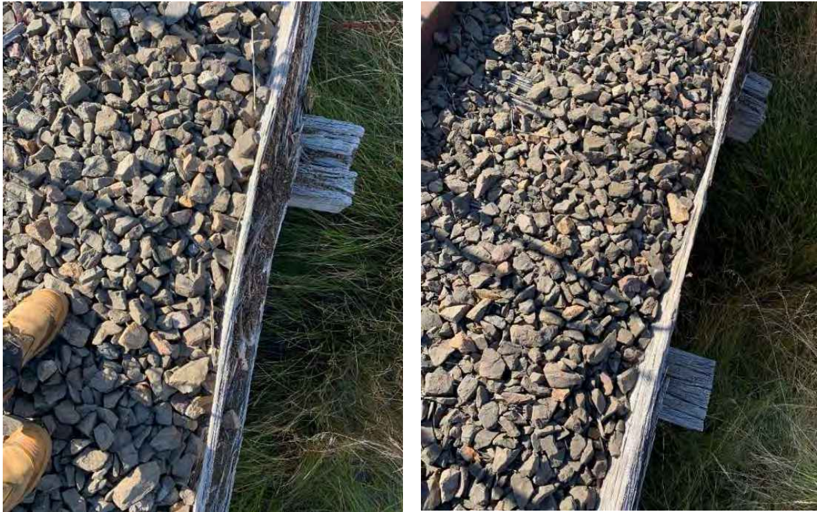
Figure 7-6: Above photos show a ballast tray side wall lengths that have completely rotted away, significantly reducing its ability to retain the ballast material.
