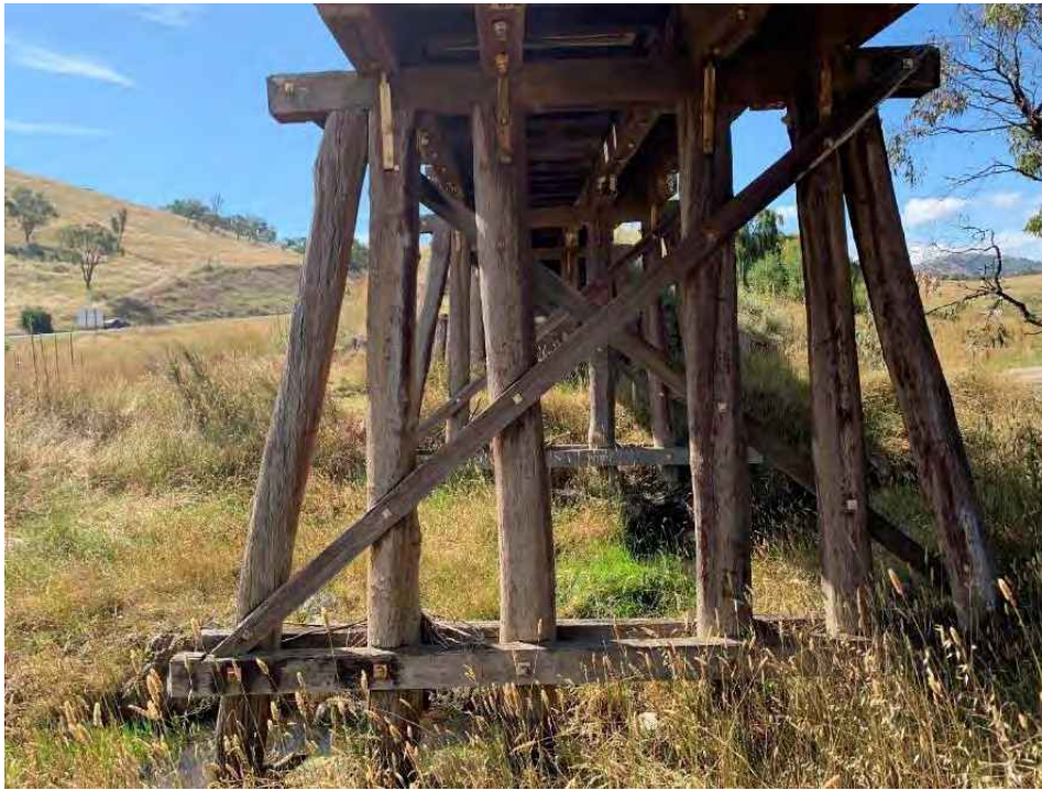
Figure 8-2: View of the typical timber pile bents configuration. The bents comprise of 6 driven piles (4 Plum piles directly under the girders and 2 batter piles on either side). Pile bent 2 and 3 are supported by cross bracing and timber wales at the bottom of the bent. Pile bent 3 was constructed on a concrete footing. The two abutments do not contain the cross bracing and wales. It was noted that the bottom section of several posts and timber cap wales have started to undergo decay. This can be expected due to the timber posts bearing directly on the concrete footing which typically has a high moisture content. Over time the timber post undergoes capillary action and draws up the moisture like a ‘straw’. Once the moisture content in the timber elements reaches 22%, decay causing fungi are activated and the decay process begins. Overall, the timber bents were found to range from fair to very poor condition.
