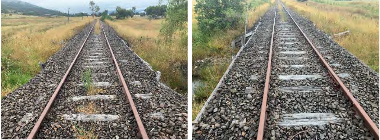
Figure 5-8: Top view of rock ballast looking in opposite directions. The rock ballast was found to be in fair condition with no major erosion present, no holes were found in bridge decking. Transoms were found to be in fair to poor condition with moderate deterioration and decay found.
