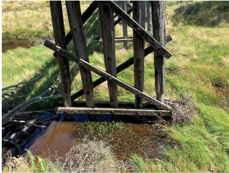
Figure 10-3: Significant decay is present on all piles in above image. Large decrease in pile cross-section on the bottom end of the piles located in the river (Body of water). Debris is caught up in the wales and surrounding areas of pile bents. It is recommended that deteriorated sapwood be removed appropriately.
