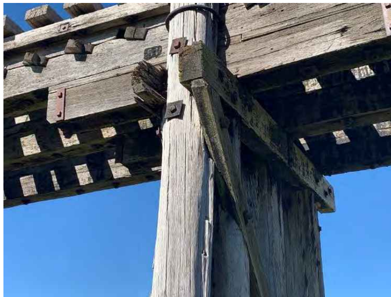
Figure 9-4: The images above show the condition of the split headstocks. The majority of headstocks were found to be in poor to very poor condition. The left member in the image above is completely decayed through the end and in very poor condition.
