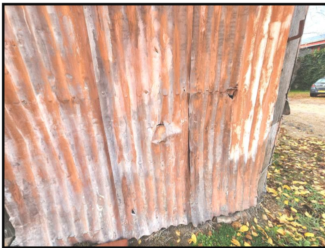
Photograph 30 Holes & corrosion in wall cladding allows water entry. No cladding at corner
