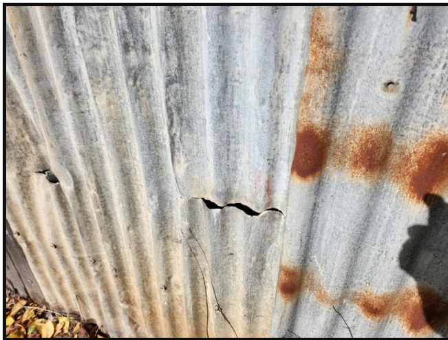
Photograph 28 Holes in wall cladding allows water entry
