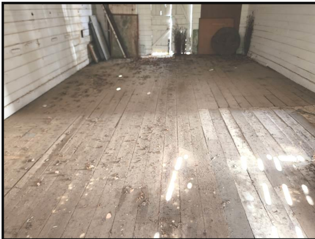
Photograph 19 Timber floor to East Wing Floor framing below the flooring is a major structural component
