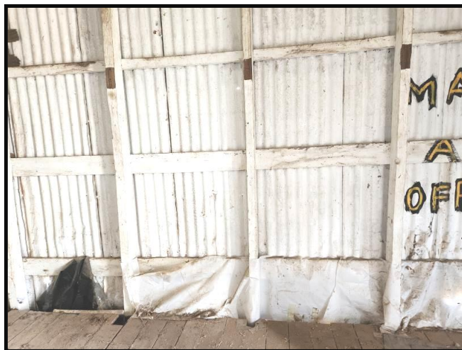
Photograph 10 No noggings between wall framing studs. The studs are excessively spaced. Wall framing is a major structural component
