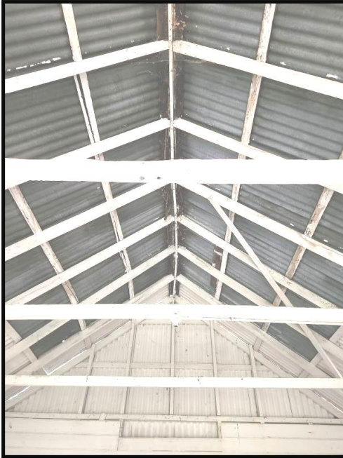
Photograph 5 Decay and sagging to the ridge at the East Wing Roof batten split Roof framing is a major structural component
