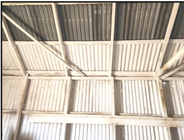
Photograph 7 Roof battens are 25mm thick & the span between rafters are approximately 920mm. Bracing does not extend to the top wall framing plate Roof framing is a major structural component
