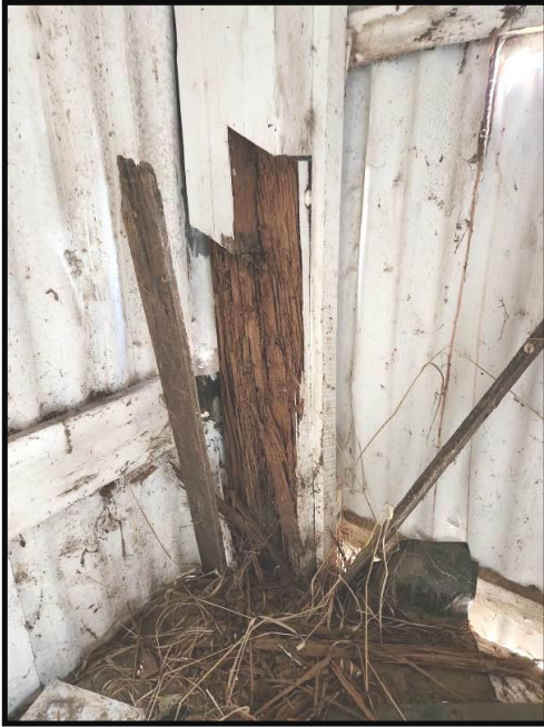
Photograph 14 Termite damage to timber post at south west corner of the West Wing. This post is in two pieces. Wall framing is a major structural component
