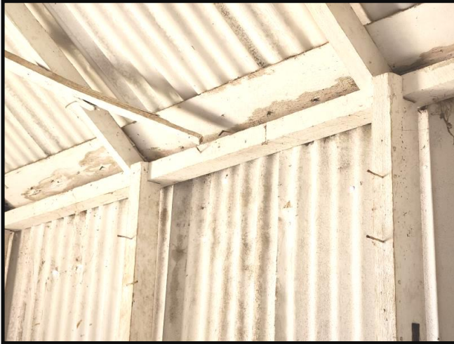
Photograph 11 Excessive notching at studs Wall framing is a major structural component
