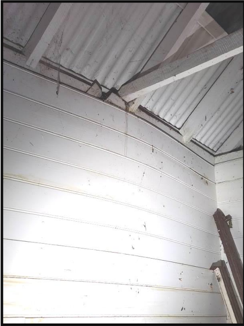
Photograph 18 Bowed wall at south east side of East Wing, due to heave from tree Wall framing is a major structural component
