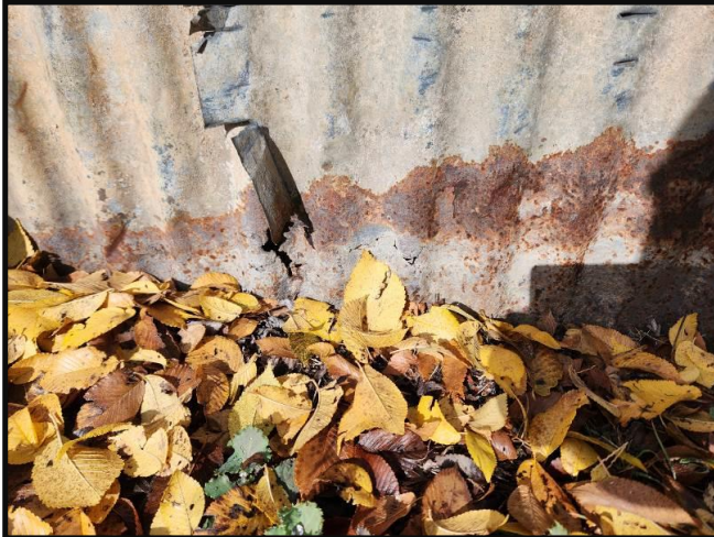
Photograph 29 Holes & corrosion in wall cladding allows water entry
