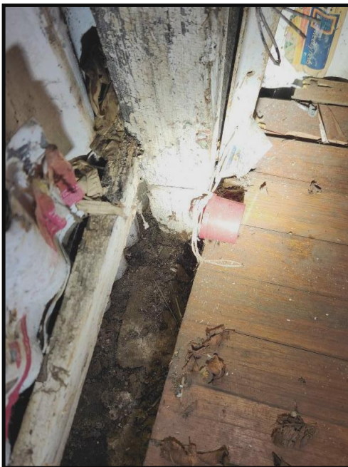
Photograph 9 Bottom plate & post in direct contact with the ground Wall framing is a major structural component
