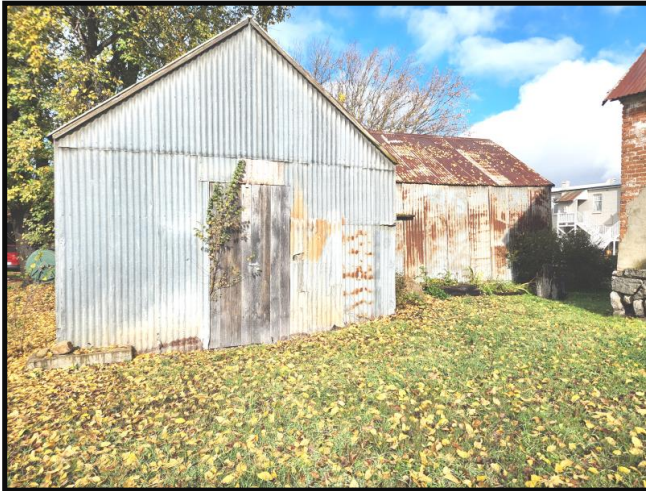
Photograph 1 Shows the front or North sides of the East Wing (left hand side) and the West Wing (right hand side)
