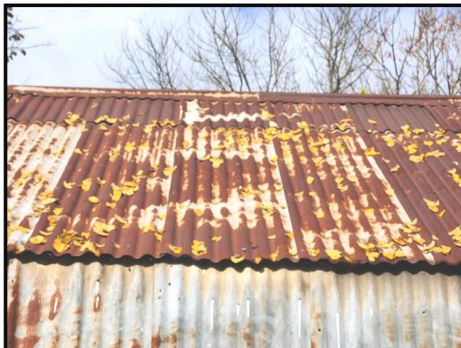
Photograph 23 Roofing to West Wing corroded, holed and not in continuous lengths
