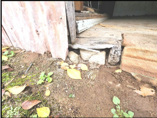
Photograph 21 Timber floor framing in contact with the ground/soil & no sub-floor ventilation to West Wing, Note wood decay. Floor framing is a major structural component
