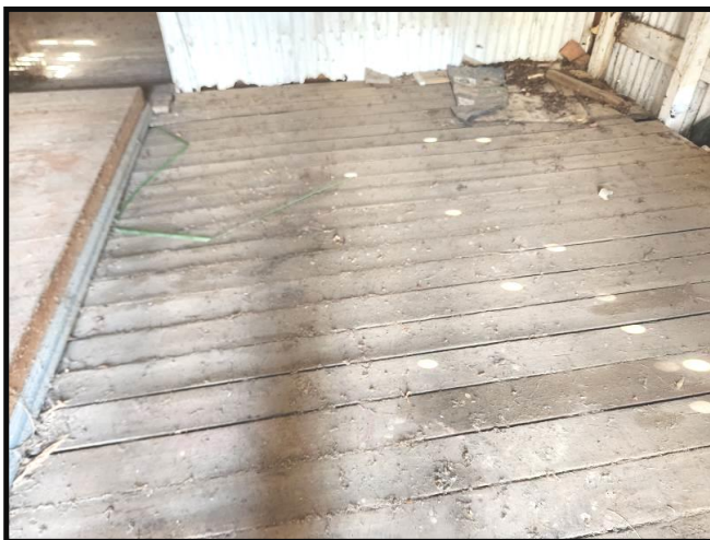
Photograph 20 Timber floor to East Wing Floor framing below the flooring is a major structural component
