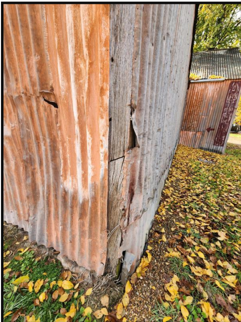
Photograph 31 Holes & corrosion in wall cladding allows water entry. No cladding at corner
