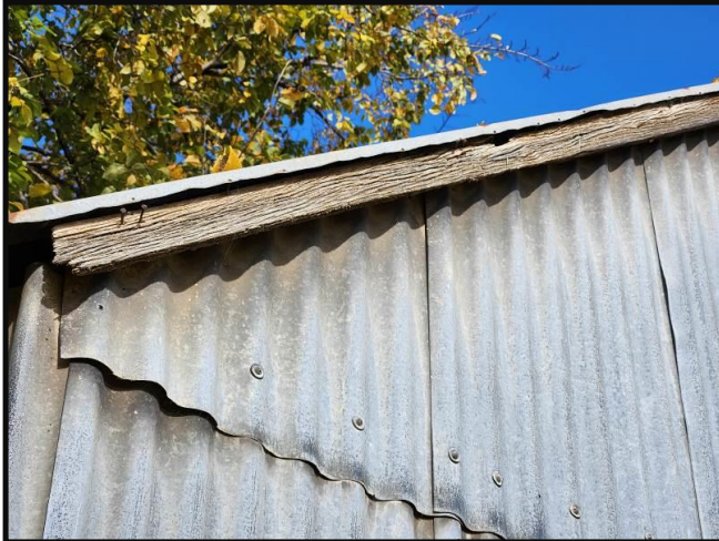
Photograph 24 Decay to fascia, indicative throughout
