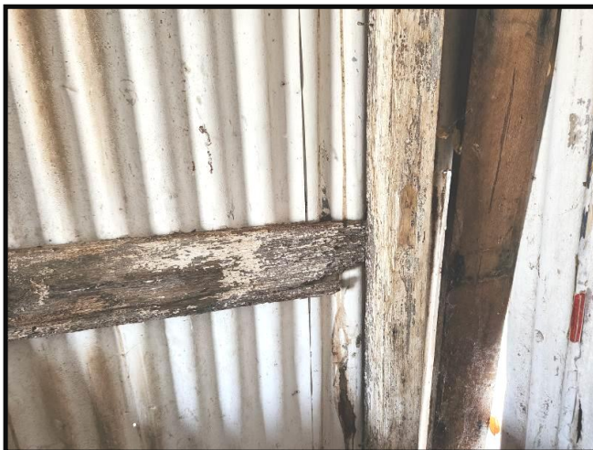
Photograph 13 Wood decay at wall batten
