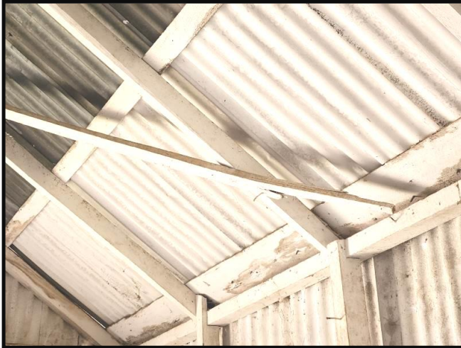
Photograph 8 Roof battens are 25mm thick & the span between rafters are approximately 920mm. Bracing does not extend to the top wall framing plate Roof framing is a major structural component
