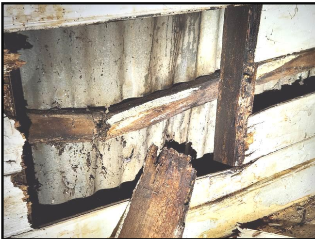
Photograph 17 Damage & wood decay at south east corner of the East Wing, due to heave from tree
