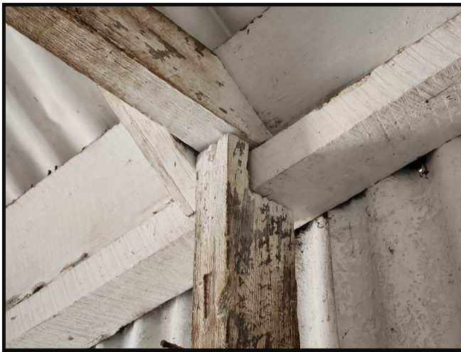
Photograph 12 Excessive notching at wall stud Wall framing is a major structural component
