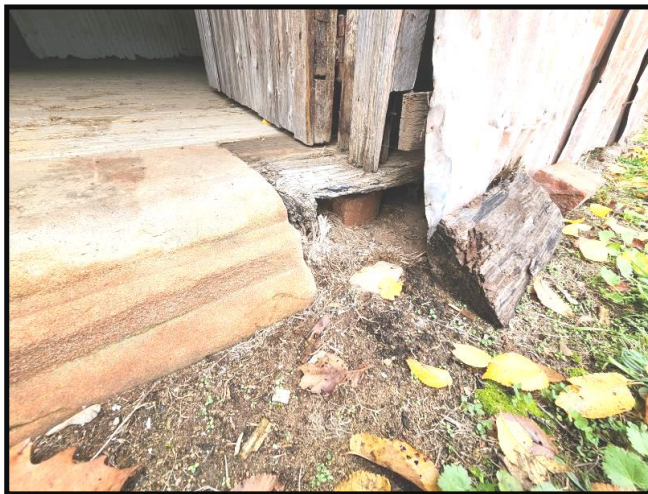
Photograph 22 Timber floor framing in contact with the ground/soil & no sub-floor ventilation to West Wing, Note wood decay. Floor framing is a major structural component
