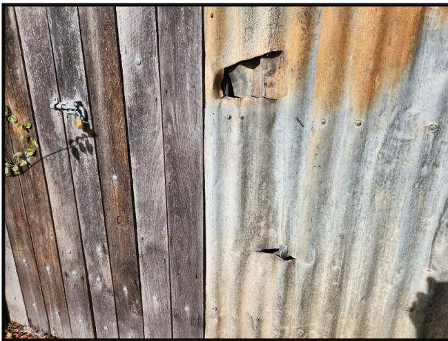
Photograph 27 Holes in wall cladding allows water entry
